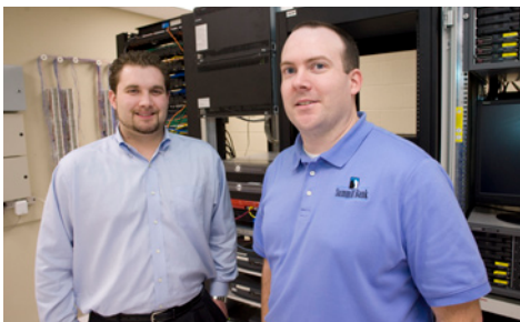
Justin Rhymes of Summit Bank and Ryan Flynn of NSG, at left, designed the Toshiba CIX telephone system that meets the bank's goals of maximizing customer service and improving inter-branch communications.
