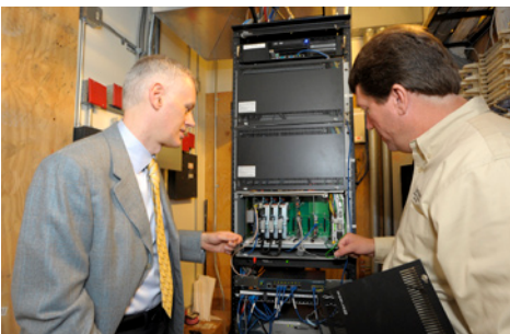
David Shapendonk of IMAX, at left, and Ben Berg of Transcom, check out the Toshiba Strata CIX in IMAX's telephone room.
