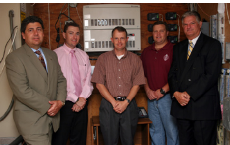
The University Christian School Toshiba system consists of a Strata CIX670 system with 208 ports that serves the school's 150+ employees and 900+ students.
